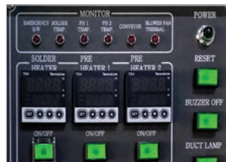
Simple manipulation allowing an entire view of the control system at a glance (Analog type error monitor)
